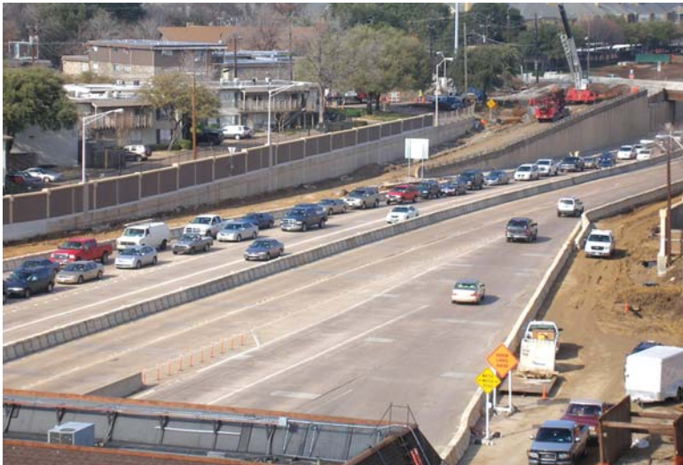
Looking north from the Wycliff Plaza during construction. With many of the toll collection lanes closed, traffic snarled and congestion stretched for miles
